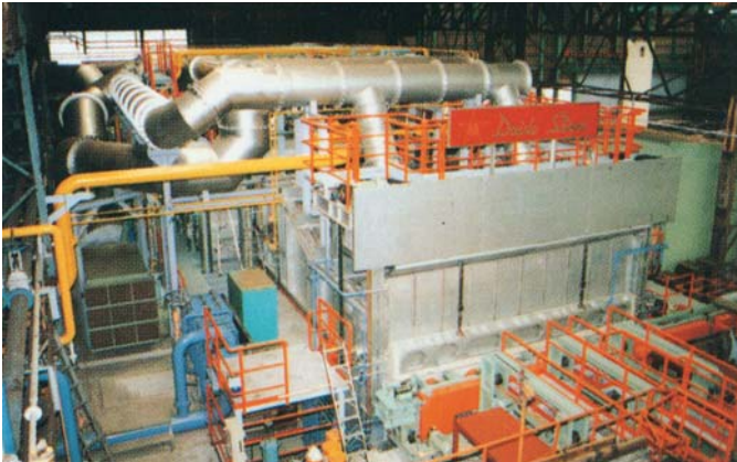
加熱炉 Reheating furnace
