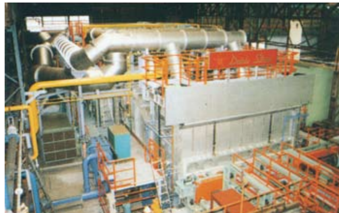
加熱炉 Reheating furnace
